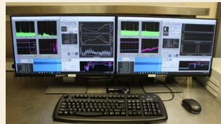
Communications Control System
